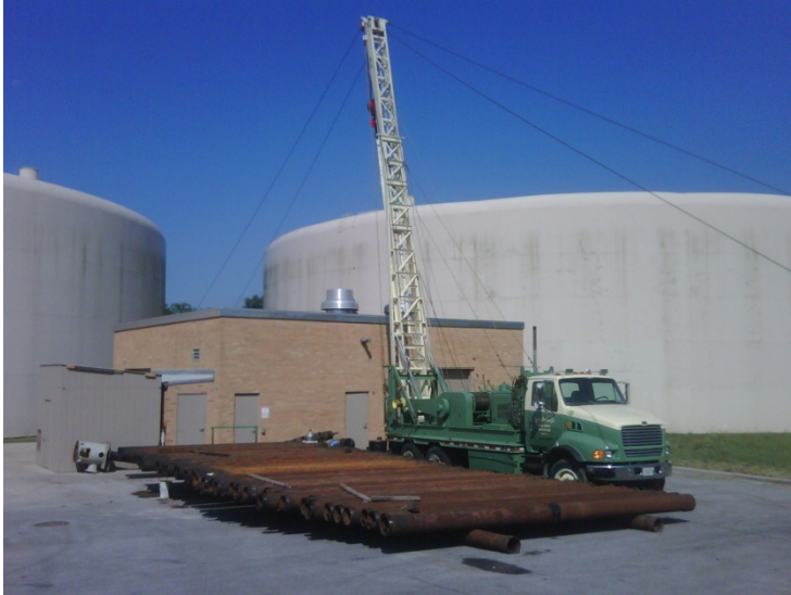
Layne used a pump service rig to remove an oil lubricated pumping assembly set to a depth of 1,000 ft. and weighing 80,000 lbs.
