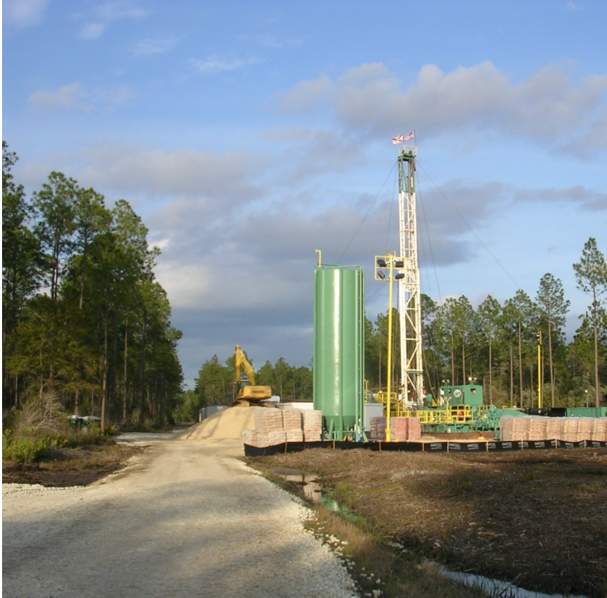
Layne drilled 24-hours per day, 7-days per week to reach 6,000ft. below land surface.
