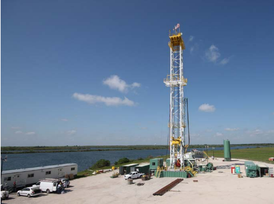
Layne worked 24 hours per day, 7 days per week to drill to 8,000 feet below land surface.
