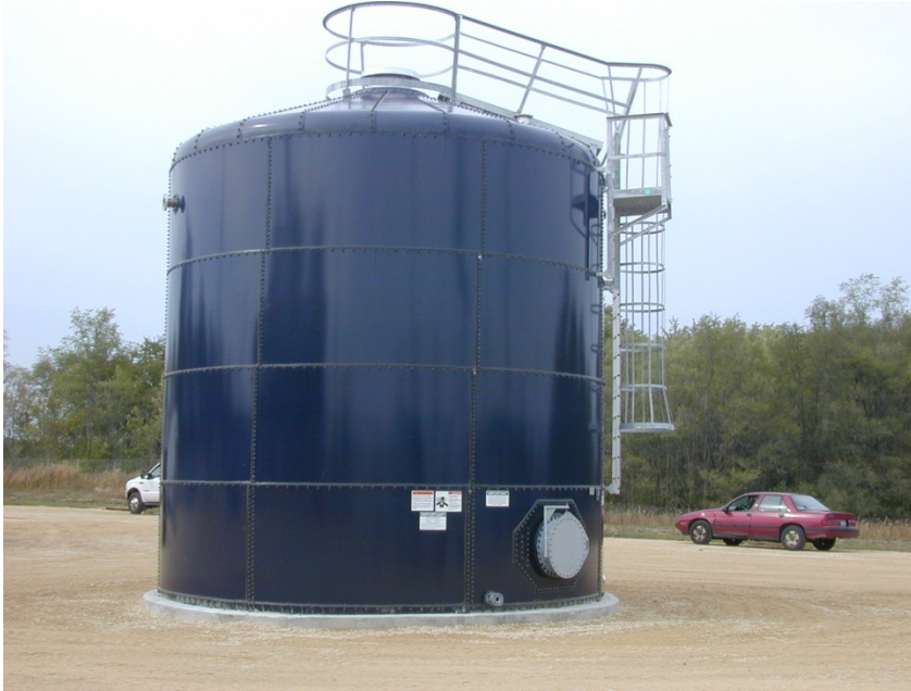
Layne completed a design-build water supply system for an industrial facility in southeastern Wisconsin with a tight schedule including all related permits.
