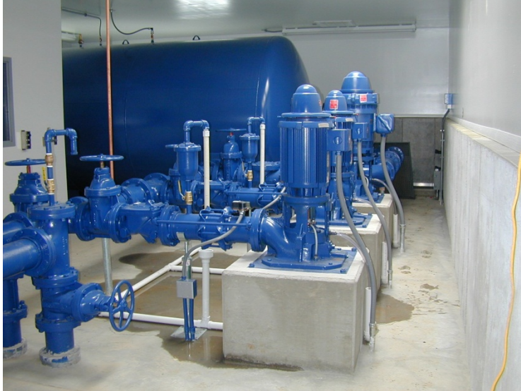
Layne was hired by the developer of a new subdivision to design, permit, and construct a community water system with a very aggressive time schedule.
