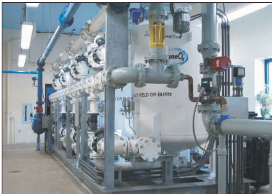
This Johnson Creek, Wisconsin 500 gpm capacity water treatment plant utilizes LayneOx media to remove water contaminants efficiently and economically.
