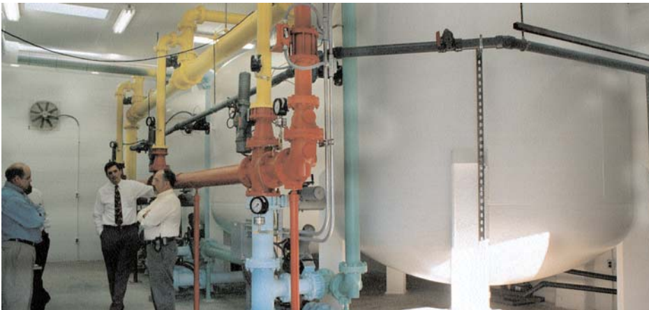
Well #13 - Ion Exchange Unit
