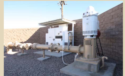
Variable frequency drive (foreground) Well & pump control panel (background)
