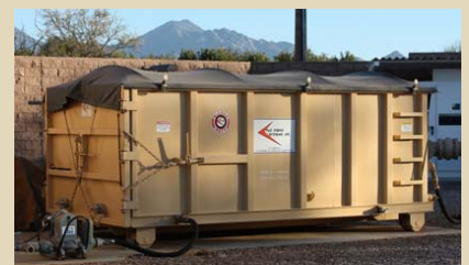
Sludge Densification Unit dewateres the arsenic sludge before disposal.
