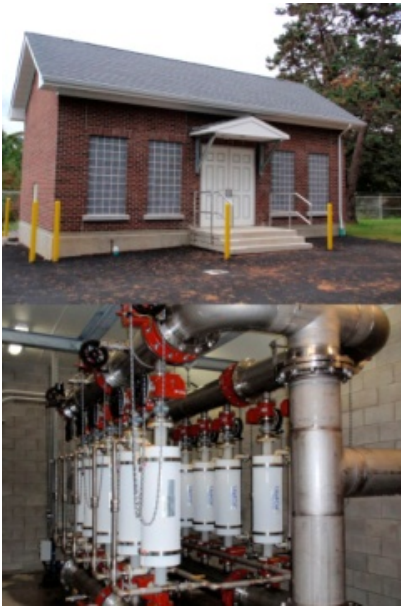
Membrana Liqui-Cel deaerators remove entrained air at the UWN treatment facility.
