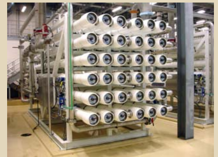
Shown above is one of four RO trains, each capable of producing up to 1.5 MGD of pure water.
