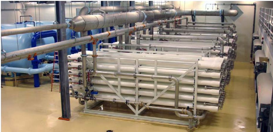
Interior of this Hutchinson, Kansas treatment plant shows Reverse Osmosis trains.
