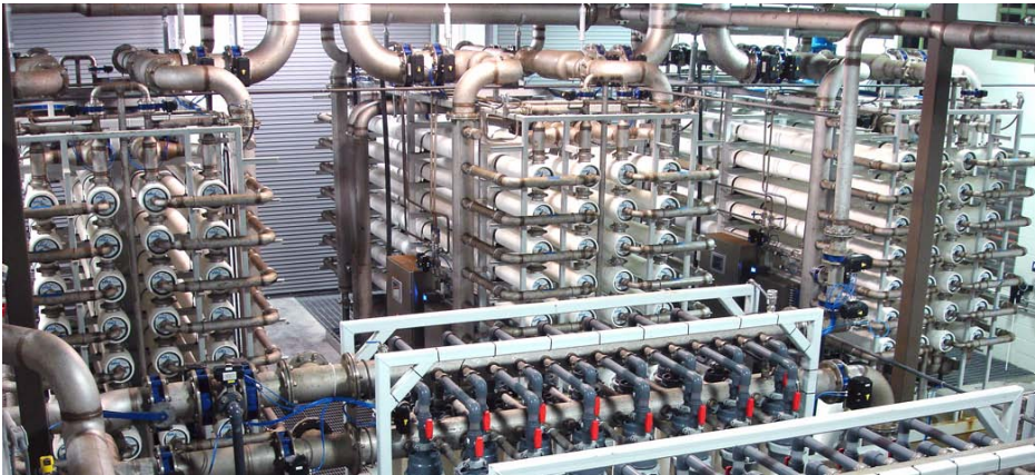
Palatka UF plant showing 6MGD Norit XIGA trains in background (horizontal elements) and 1MGD Norit Aquaflex trains in foreground (vertical elements).
