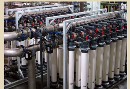
1MGD Norit Aquaflex secondary UF skids provides backwash waste treatment to increase system recovery.
