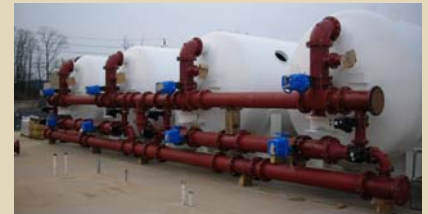
Dual train multimedia pressure filters.
