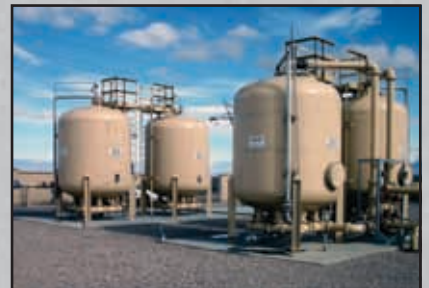
LayneRT arsenic removal system installed for Sahuarita Water Company in southern Arizona.
