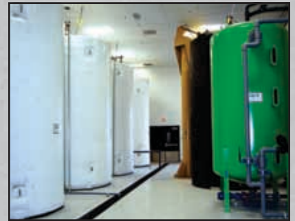
The LayneRT Media Regeneration Facility located in Phoenix, Arizona.
