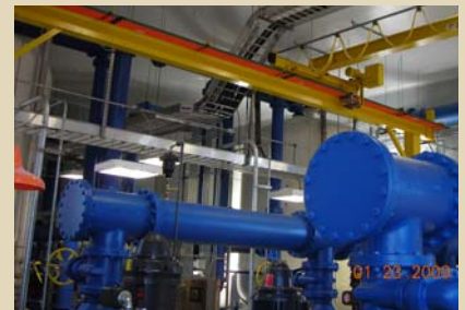
Interior view of completed facility process piping.
