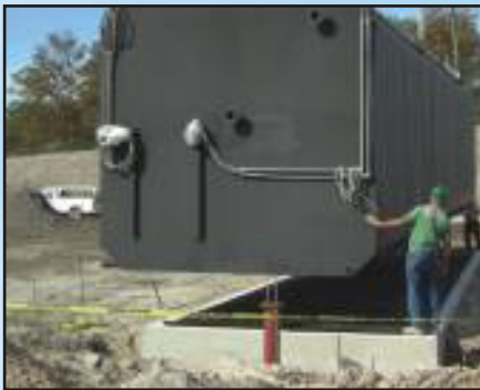
A Layne crew installs a packaged wastewater treatment plant (Fluidyne ISAM SBR) in Lewes, Delaware.
